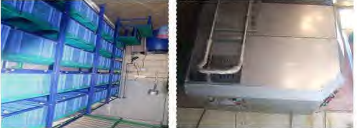
A View of Organic Waste Converter & curing system installed @ Gateway Park, Mumbai
